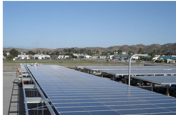
Elsinore Valley Solar Panel Alternate 807
