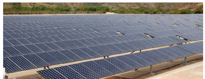
View of Hill Canyon WTP solar panel array.
