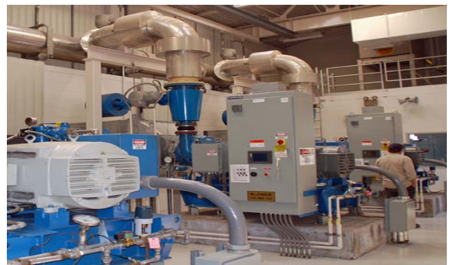
Hill Canyon WTP's high efficiency blowers.
